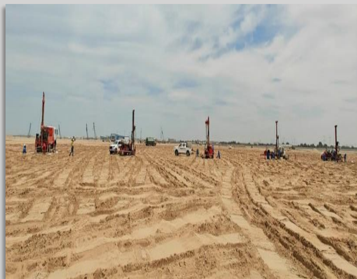
5 AHSL GT rigs working in tandem at a site in Abu Dhabi.
